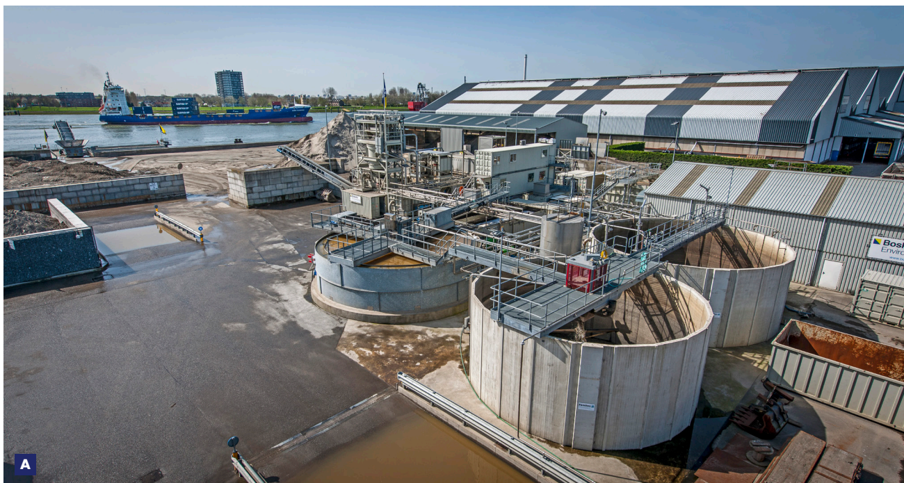
A Soil treatment installation in Schiedam
