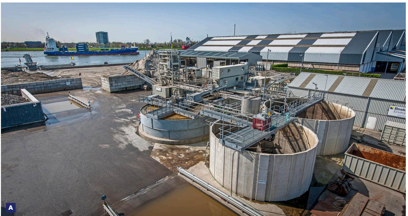
A Soil treatment installation in Schiedam
