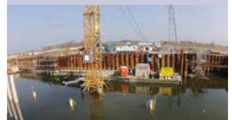
| Overview of flooded Muiden aqueduct
