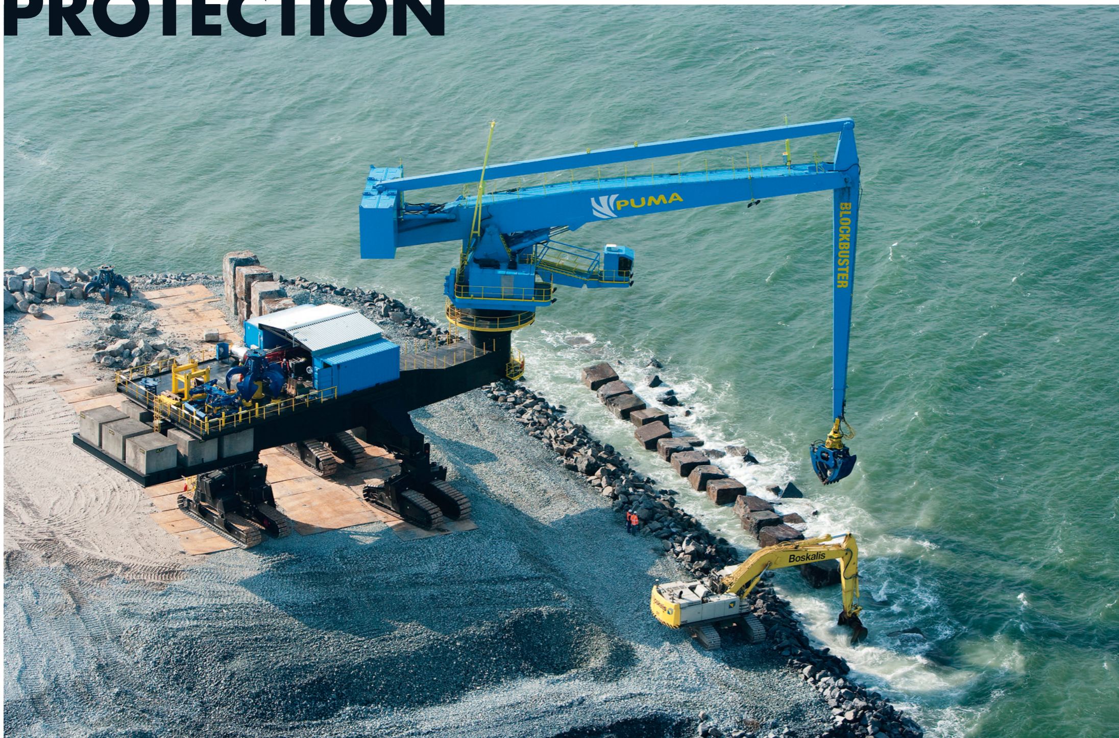
ROTTERDAM, THE NETHERLANDS The E-crane 'Blockbuster' was designed to build the sea defense of the Maasvlakte 2 port expansion. Its innovative construction enabled it to lift 50 ton blocks and accurately place them 60 meters away.
