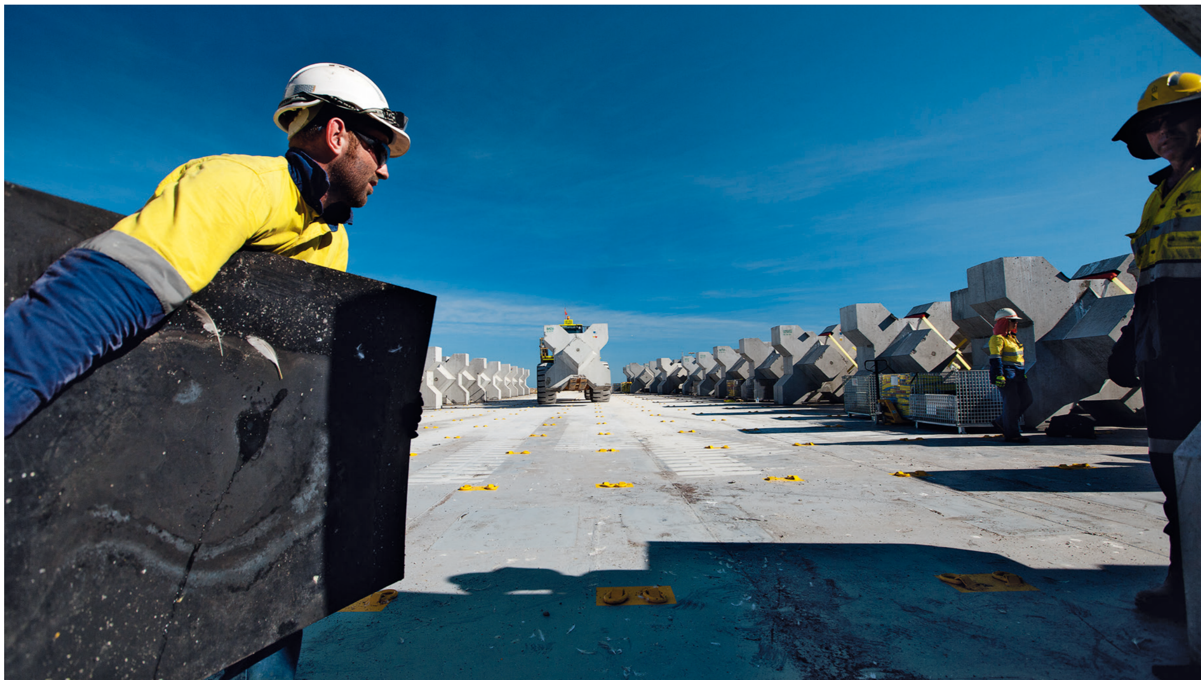
BARROW ISLAND, AUSTRALIA Design and construction of a material offloading facility, a roll-on-roll-off facility and 200m of quay walls.
