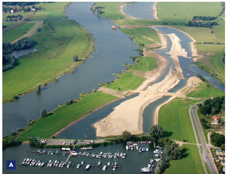
A Deventer Project: aerial view of the work in the Stobbenwaarden area.
