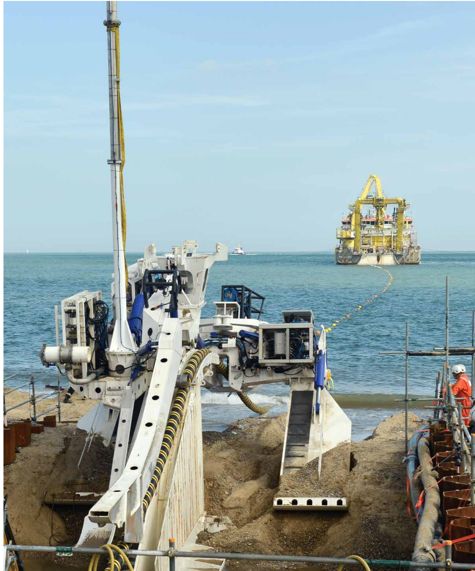
Shore landing of export cable by cable laying vessel Ndurance and HD3 plough
